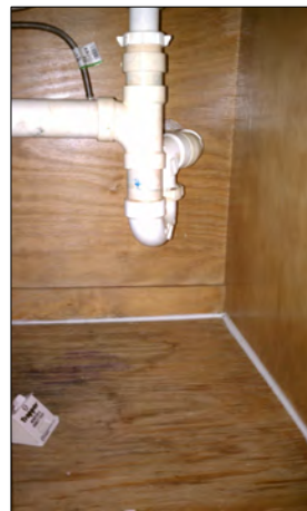
Monitor under a well-sealed sink
