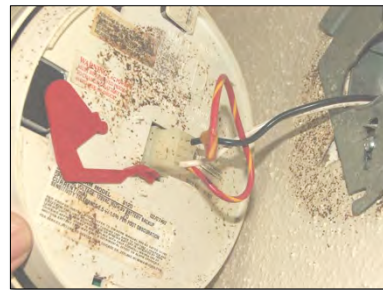
Cockroach infestation in a smoke detector
